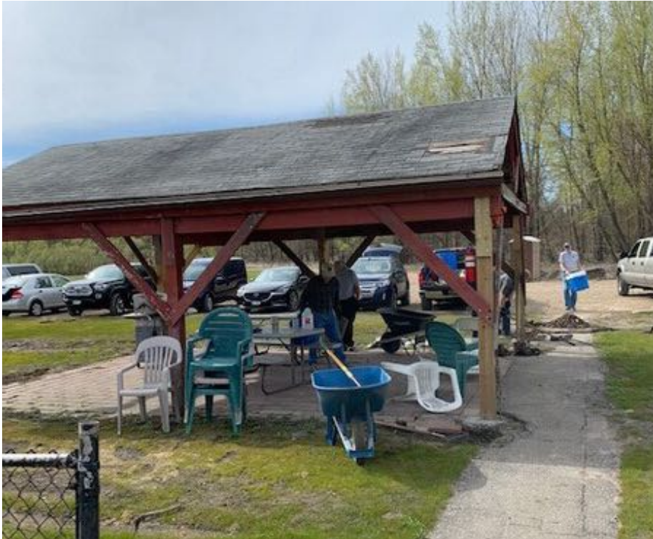
The shelter crew did a great job with the pavers and walkway. (Photo by Tim Wirtz)
