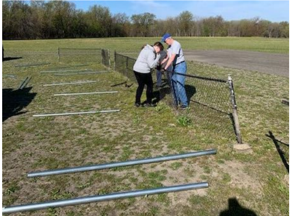
The new poles are positioned to replace the old ones as the old fencing is removed. (Photo by Tim Wirtz)
