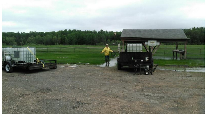
There was a lot of silt and dirt to be removed from the runways and pits.
