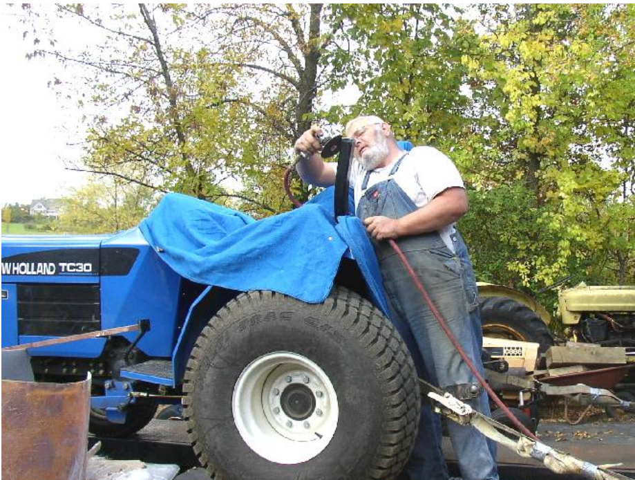
Don Knauff prepares the cut roll bar for welding. (Photo by Bill Jennings)
