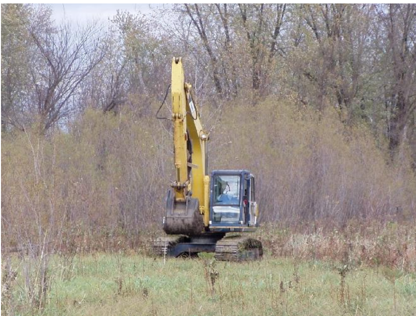
The backhoe improves the drainage to the east of the runways at the Jordan field. (Photo by Bill Jennings)
