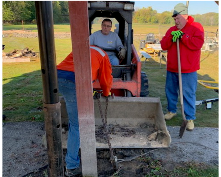
Even with the Bobcat and power auger, it was hard work for the crew. (Photo by Tim Wirtz)
