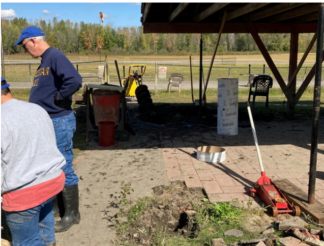
The west end of the shelter had to be supported while the two posts were removed.
