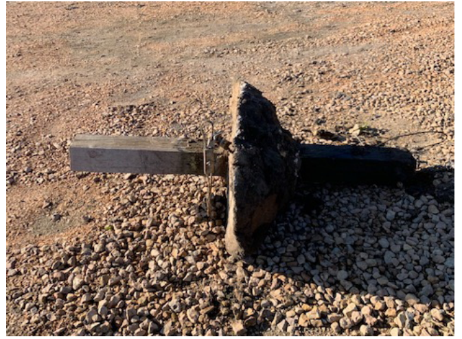
One of the old posts and its concrete after removal from the ground.
