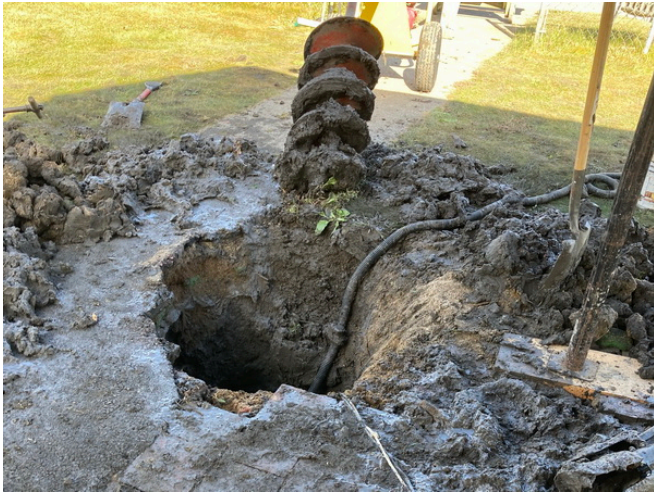
After the post and old concrete were removed, the hole was cleaned out with the power auger.
