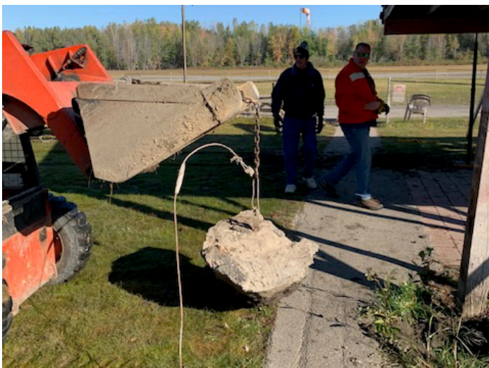
The old concrete is removed from one of the posts. (Photo by Tim Wirtz)
