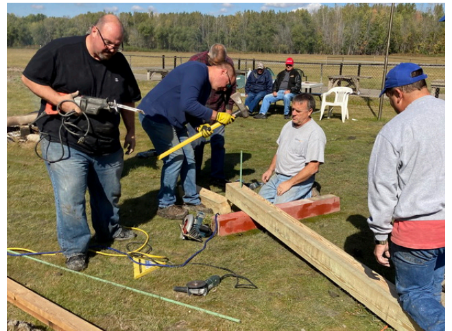
The crew readies one of the new posts for its placement under the shelter.
