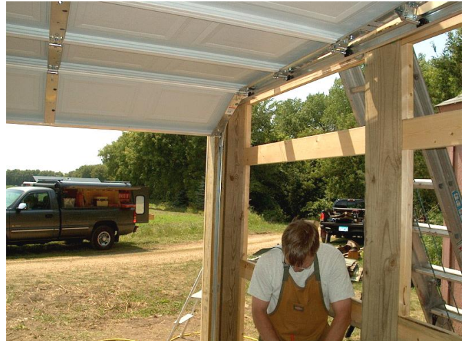
Rick Smith working on the inside of the new shed before the walls went on.
