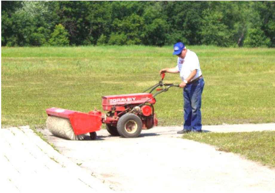
Larry Couture removes the silt on the taxiways and runways with a nifty machine. (Photo by Scott Anderson)
