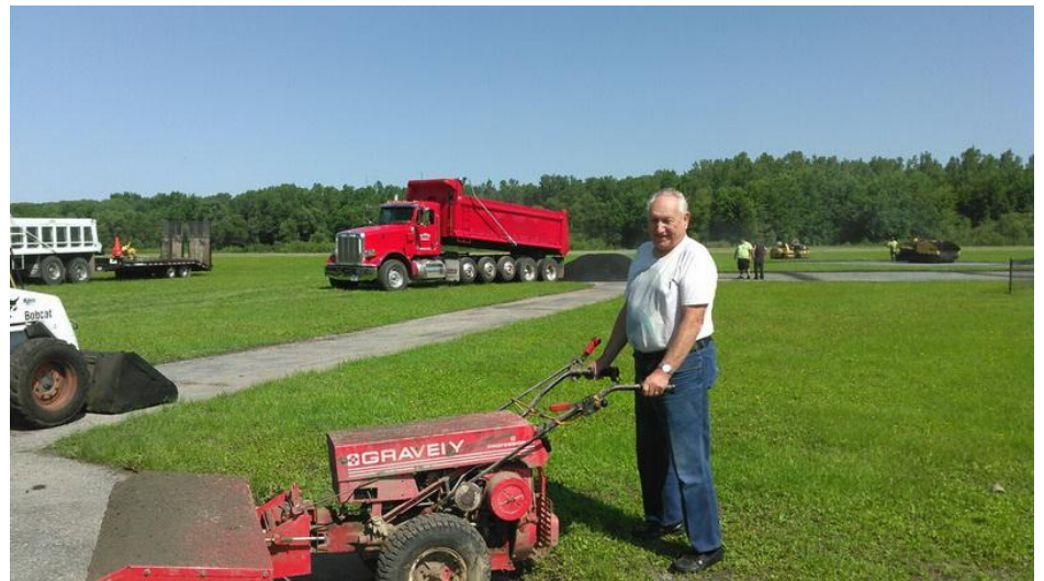
Larry Couture lends a hand during the paving of the runways. (Photo by Bob Breisemeister)
