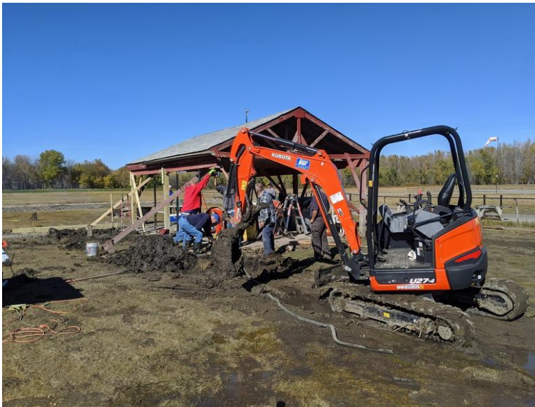
The TCRC shelter sports its new posts and foundation after all the hard work of the crew. (Photos by Tom Hall)
