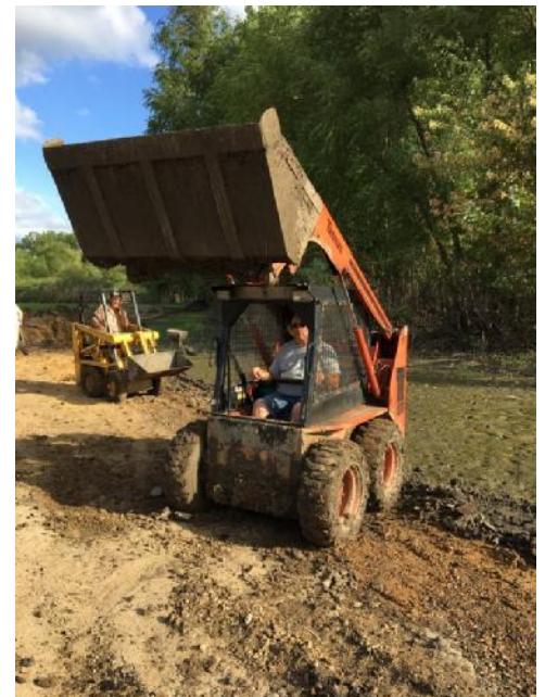
President Bob and Jim Ronhovde kept their hard-working Bobcats going constantly removing silt. (Photo by Jim Cook)
