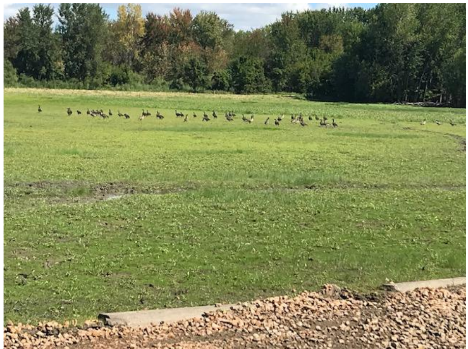
As Jim Ronhovde was busy working on smoothing the edges of the runways about 80 geese settled in to watch the show. (Photo by Jim Ronhovde)
