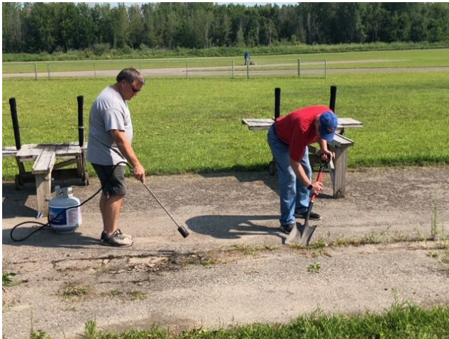
The pit area surface had to be smoothed down so that the asphalt would lay flat.
