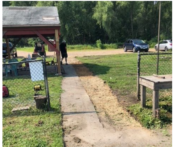
The walkway area connecting the parking lot to the shelter and pits took a lot of work.
