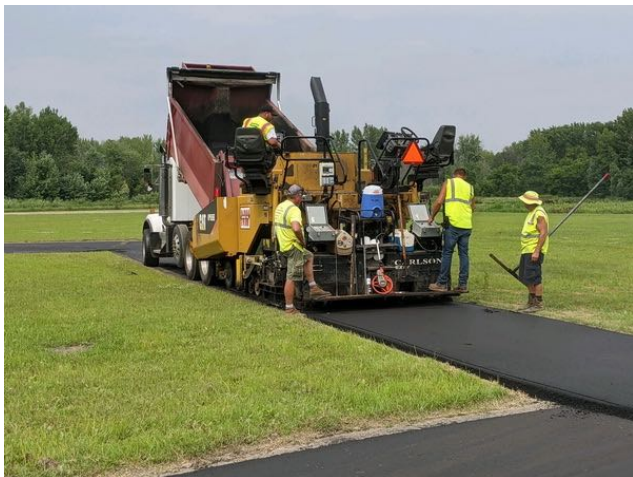
The crew using the surfacing equipment laying down the west side of the pits.
