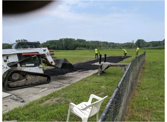
Putting the asphalt on the east side of the pits using the bobcat so the subsurface is not damaged.
