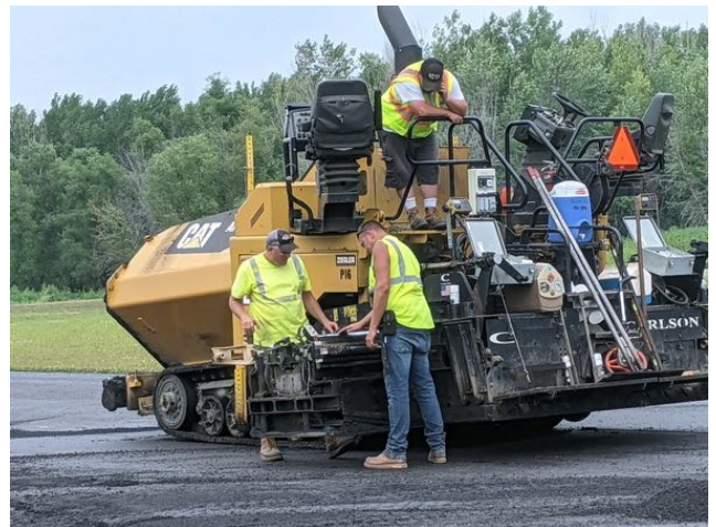
The paving equipment really did a great job of laying down a smooth layer of blacktop.
