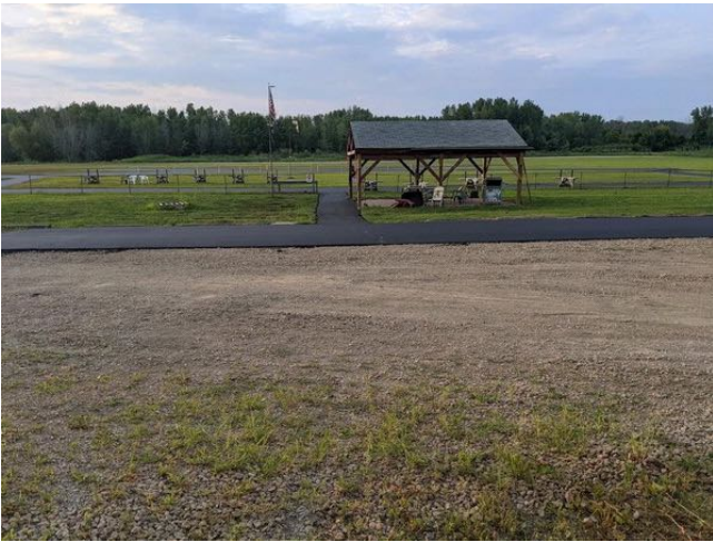
The new strip of asphalt along the north side of the parking lot and adjacent to the shelter.
