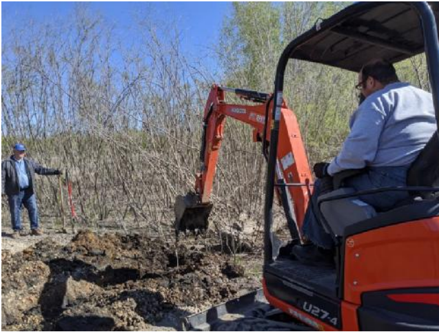
Tim Wirtz works with the backhoe to replace the culvert in the TCRC entrance road.
